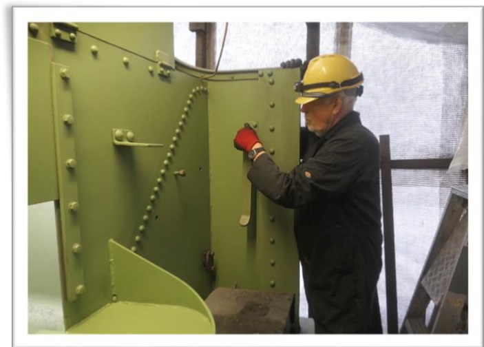
Top: View of outer wrapper of 541 firebox, with patch screws being fitted.
