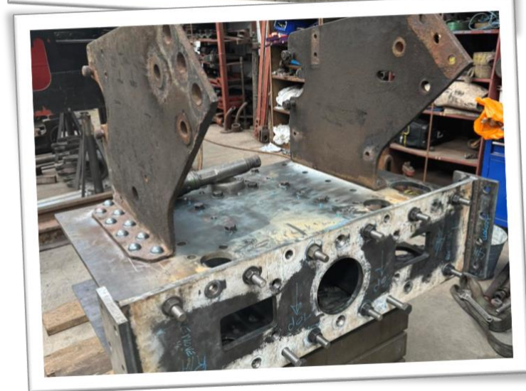
Photos, top to bottom: Copper welding on the inside of 541's firebox New machined bolts for horn blocks and a new drawbar pin Underside of new loco rear dragbox fabrication
