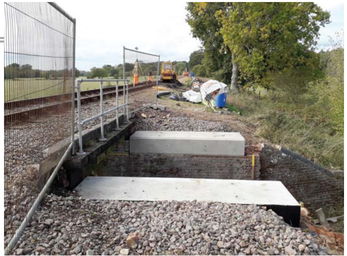
The two 1/3 sill beams fitted as the track is being lifted and laser bulldozed in the background. JON GOFF
