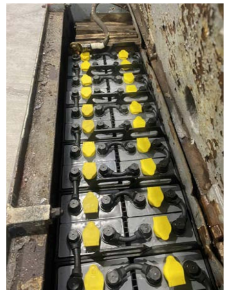
The new batteries in D4016. MIKE HAWKINS
