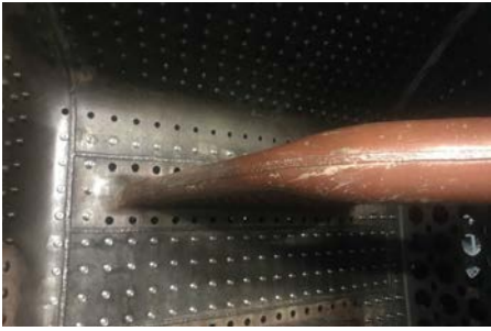
Looking up to the roof of Sir Archibald's firebox, showing the stays that remain to be fitted around the thermic syphon. TOM JAMES
