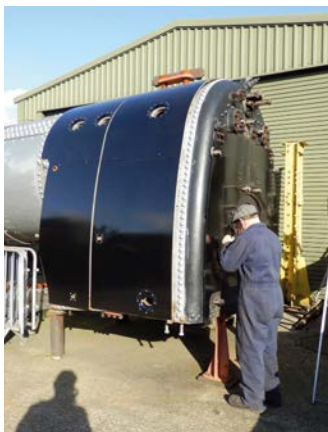
The firebox clothing sheets have sufficient paint on them to allow them to be placed in position on the boiler.
