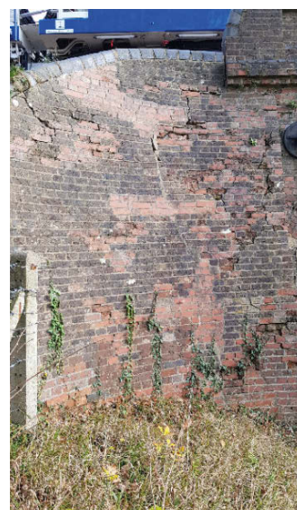
The next major project will be remedial works on New Road Bridge. VERNON BLACKBURN
