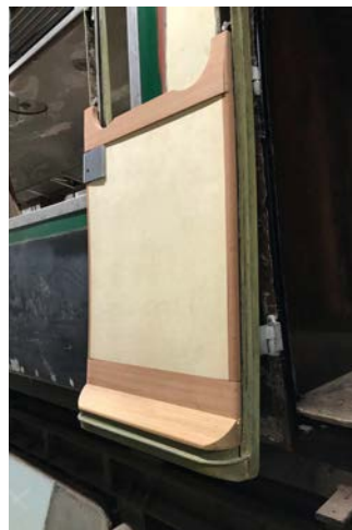
New timber door-checks are being fitted to No 4754, and then the doors are being re-hung, and fitted with new internal trim.
