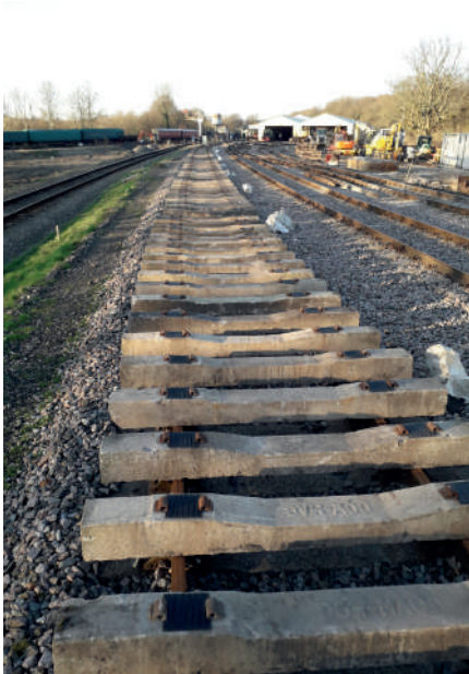
LEFT: Sleepers laid out in Horsted yard on lockdown day, ready for the Freshfield Bank relay.
