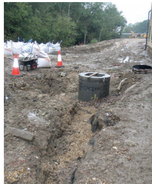
New drainage underway on the east side of the Heritage Skills Centre. BRUCE HEALEY
