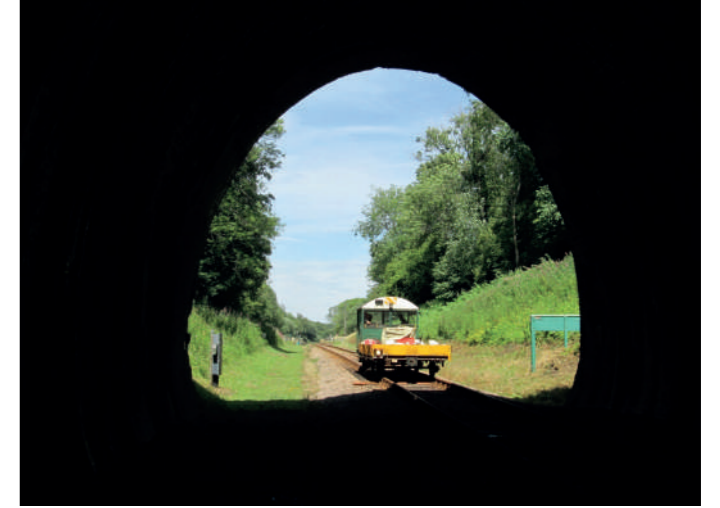
The Thursday Gang during the task of replacing rail keys inside the tunnel, many of which had deteriorated due to the damp conditions. TIM CRUMP
