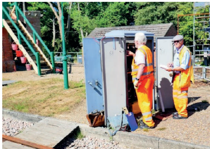
Preparing for the re-opening. Chris Chambers examines the signal equipment whilst Chris Bassett records the details. CHRIS MAJER
