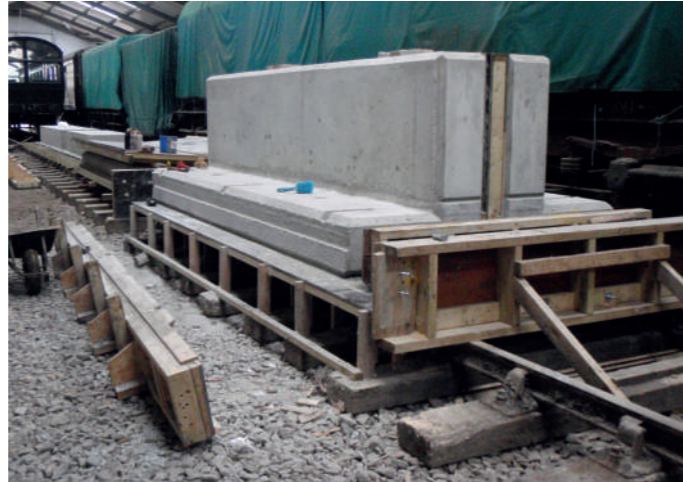
The castings for the replacement of Palmers Bridge are under way but delayed by lockdown. The sill sections, one deck section and two deck sections with parapets have been cast. BRUCE HEALEY
