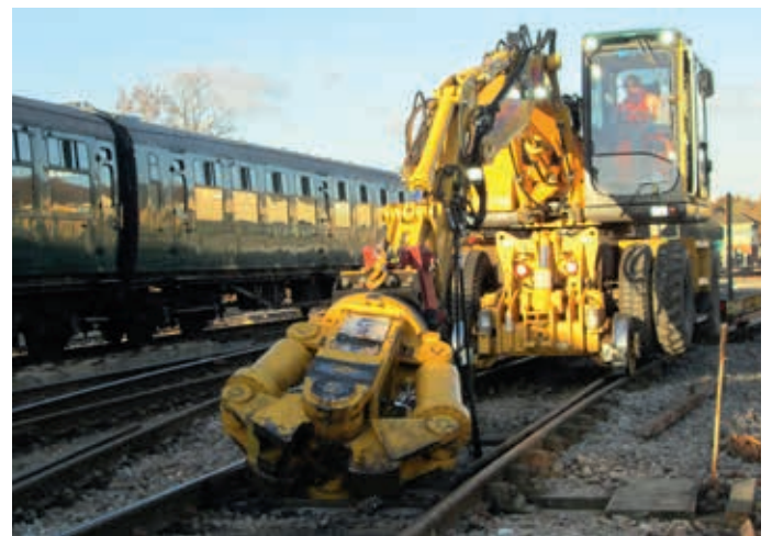
Hydraulic rail cutter on Darren's road railer snipping through old rail. TIM CRUMP
