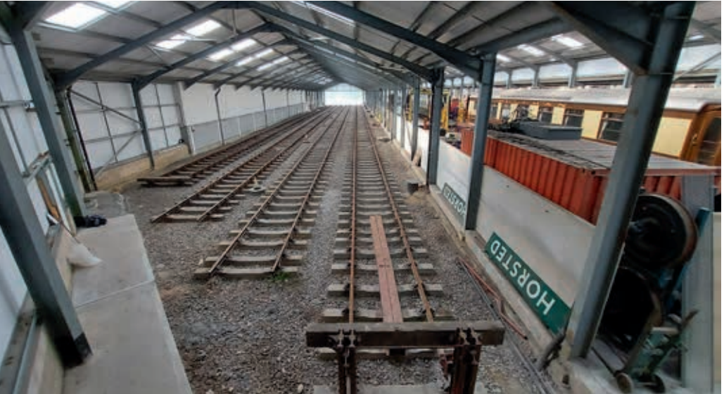
A view of OP4 from the top of the new switch room. JON GOFF
