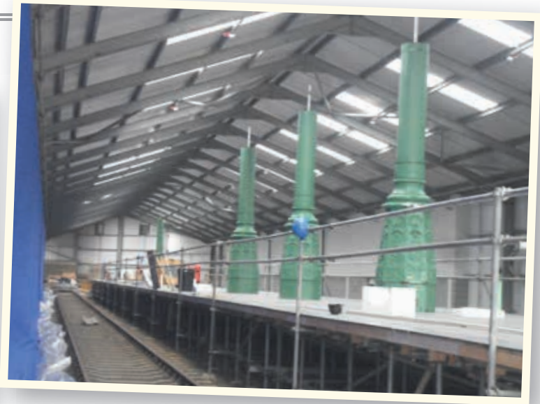
The Gare du Nord platform under construction in the OP4 carriage shed.
