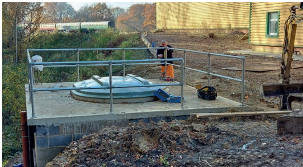
Gary Whittaker finishing of the hand rail around the septic tank. JON GOFF
