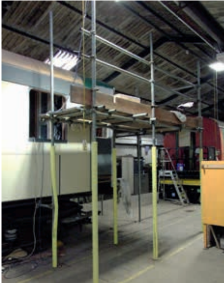
On the roof of Car 54 , following an abortive attempt to create a formed copper end cap by external contractors, the decision has been taken to create a GRP covering for the complex end shape, to which purpose scaffolding, seen here, provides access.
