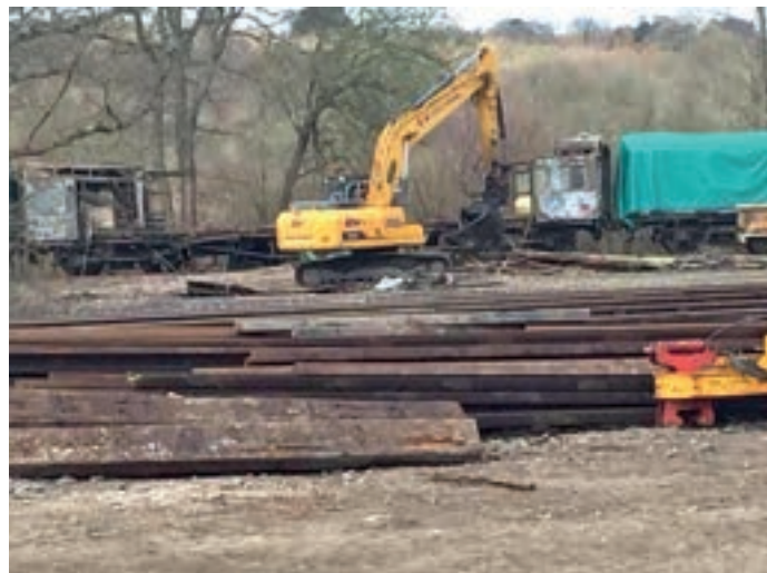
One that didn't make it: having removed all useful components, SR Maunsell Brake No 4444 succumbed to the digger's arm in April.
