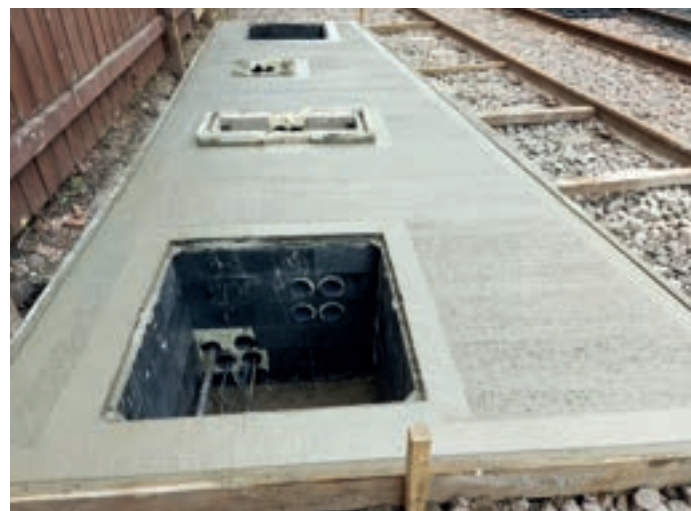
New manholes and location box bases at East Grinstead, in preparation for signalling the area. JON GOFF
