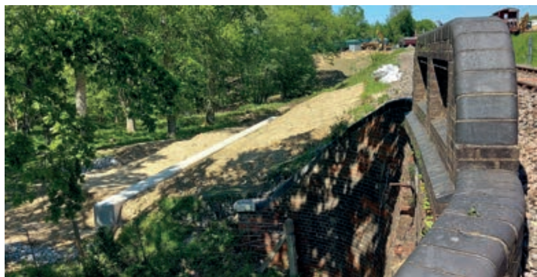
Almost buried: The retaining wall at New Road Bridge. JON GOFF
