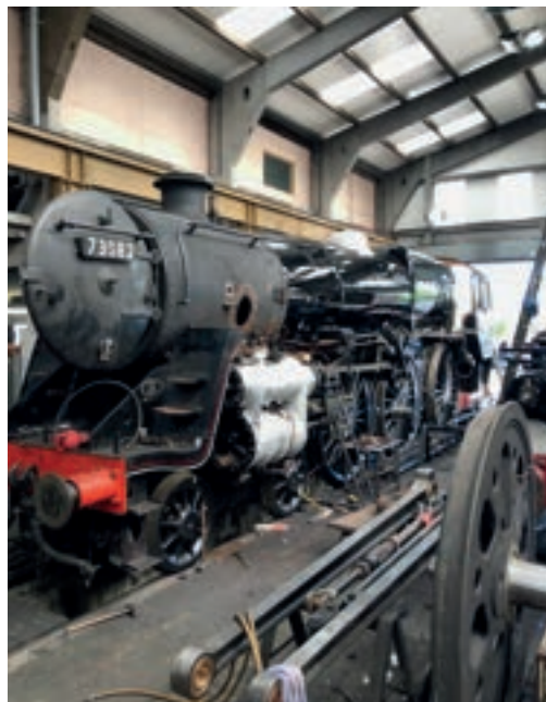
Camelot's boiler reinstated. HENRY MOWFORTH
