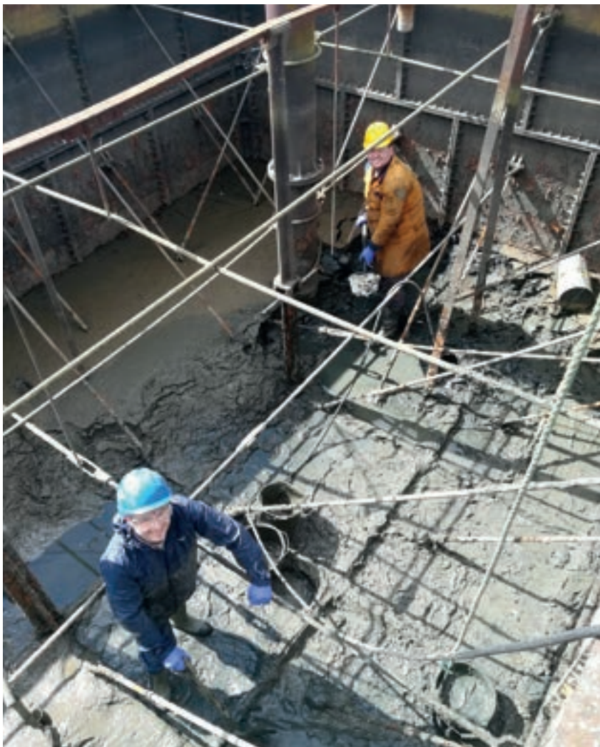
Clearing accumulated mud and silt inside the water tower at Sheffield Park. GREG WALES
