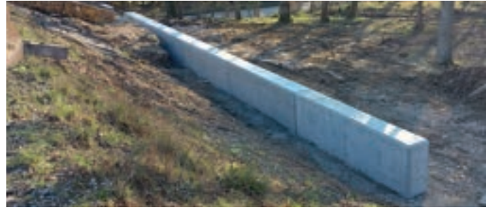
The completed retaining wall at the western embankment of New Road Bridge. JON GOFF
