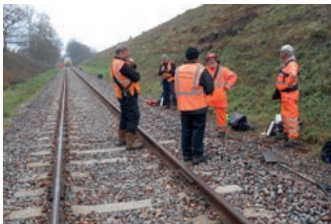
The Wednesday Gang (North) strimmer team and look-out man takes a break on 2 December 2020, while Balfour Beatty's tamper crew receive a briefing in the background. BRIAN KIDMAN
