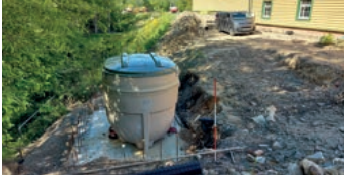
The new septic tank at OP4, prior to burying and re-landscaping. JON GOFF
