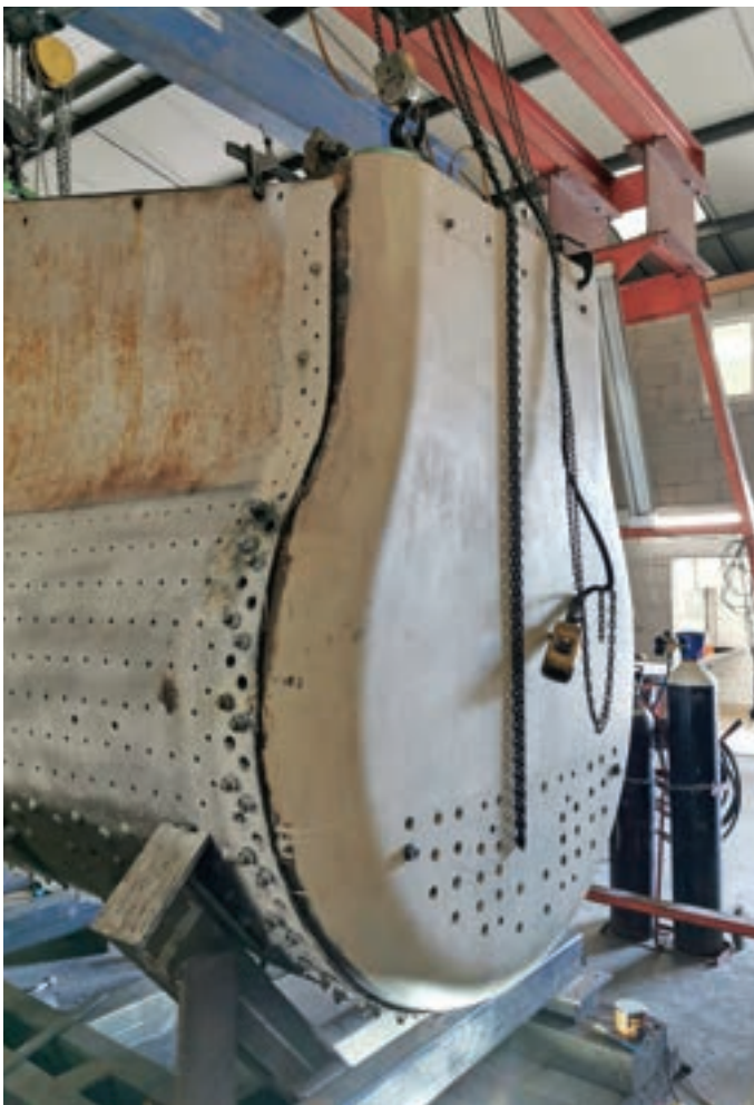
Stowe's new boiler backhead, drilled and in place ready for riveting to the steel outer firebox wrapper. HBSS
