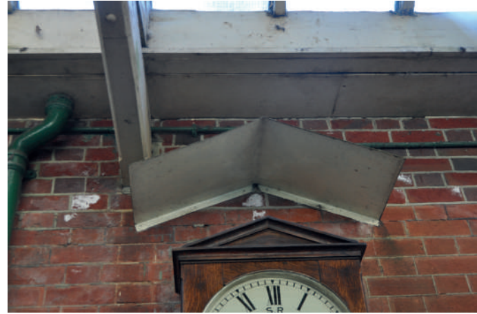
Even the station clock needs its own 'tin hat' to protect it from water running down the wall from failed flashing.
