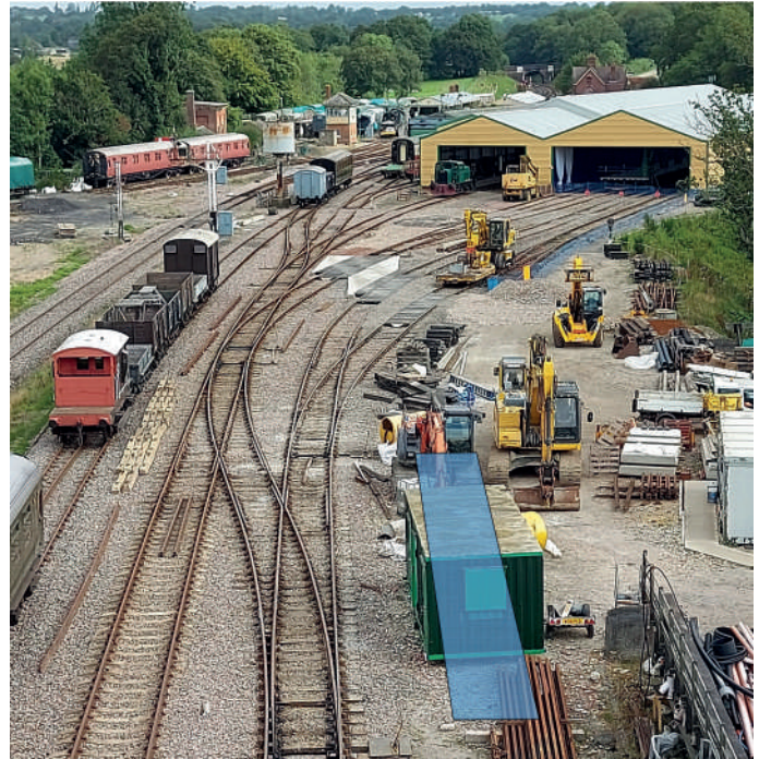
The position of the inspection pit within the rebuilt down yard. JON GOFF
