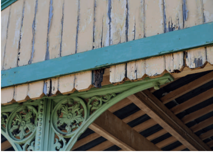
Rotting timbers on the canopy face.
