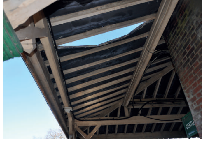
Daylight! Failed zinc sheeting at the Gents' on platform 5.
