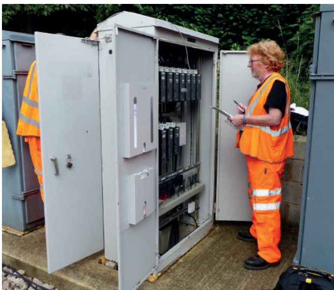
Our friends from Siemens used their volunteer days to help us set up and test the Westplex system.
