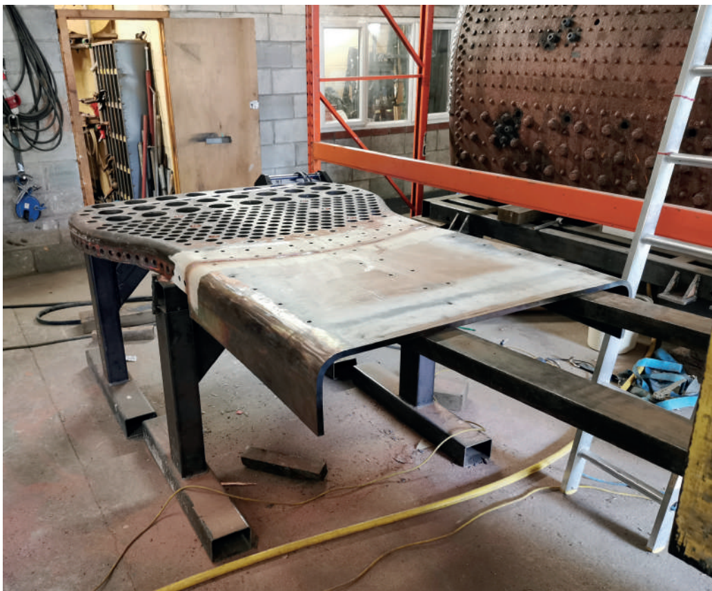
The new bottom half of the inner firebox throatplate aligned with the 'old' top half. HBSS
