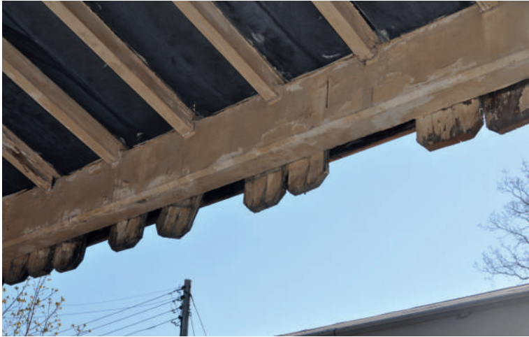
Missing teeth: Canopy valancing has suffered from water damage.
