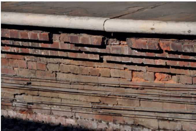
Spalled and missing brickwork on platform faces.
