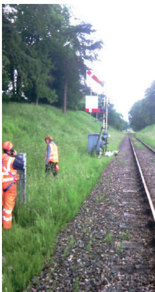
Signals 41 and 43 sighting boards.
