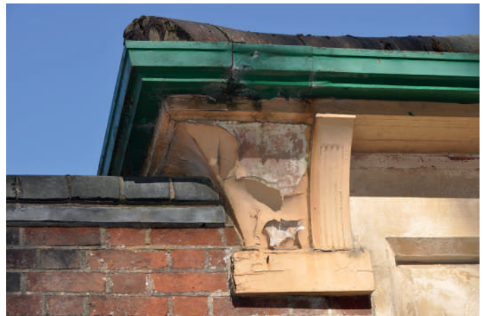
Peeling paint on plasterwork.
