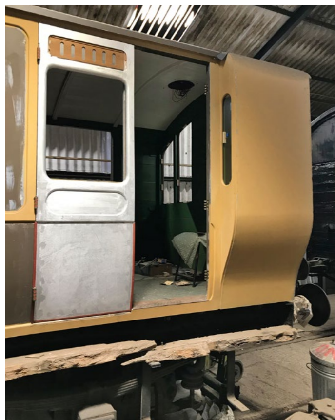
RIGHT: The majority of work on Stroudley Brake No 949 has concentrated on glazing the brake area and panelling the doors, and one of the brake doors is seen here. RICHARD SALMON
