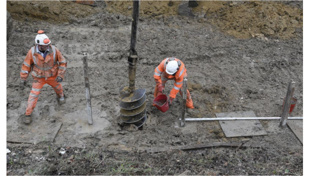
Matt Crawford and Andy Palmer with John Millam driving the auger, drilling the pile holes. JON GOFF
