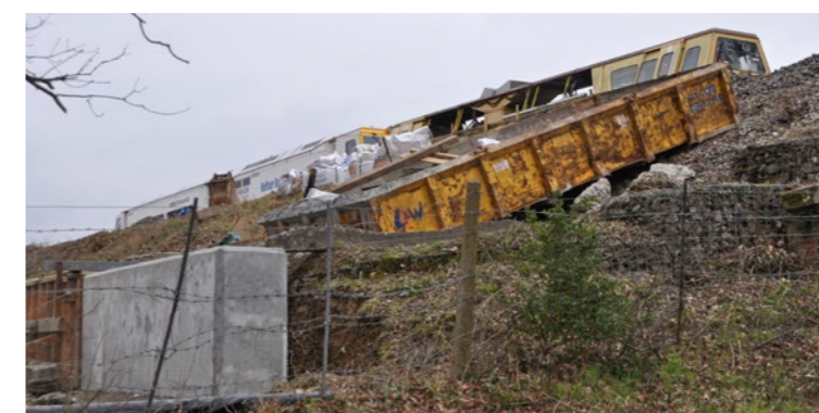
Concrete piling in place on the western embankment at New Road Bridge, Horsted Keynes. COLIN TYSON
