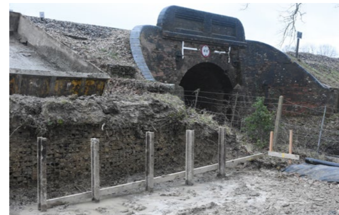
Reuse of the old rails in the retaining wall at New Road Bridge. JON GOFF
