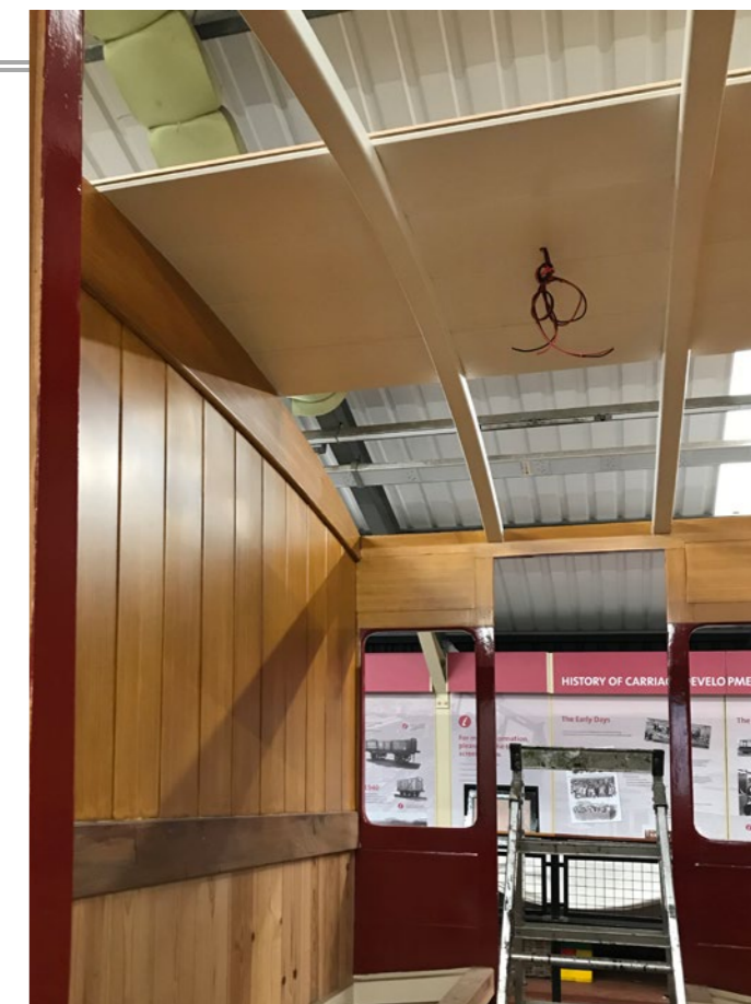
RIGHT: Stroudley/Billinton Third No 328 has had its first roof planks fitted and wiring for the lights (which will be electrically illuminated gas lamp fittings) has been run. RICHARD SALMON
