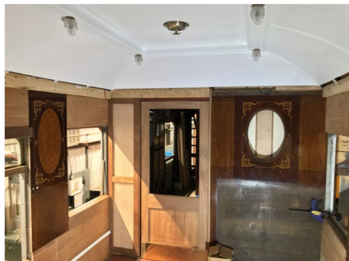
The relocated partition between the wheelchairlift entrance area and the enlarged saloon necessarily now has a wider doorway than the original, and the newly made wider sliding door is seen here prior to staining and polishing. RICHARD SALMON
