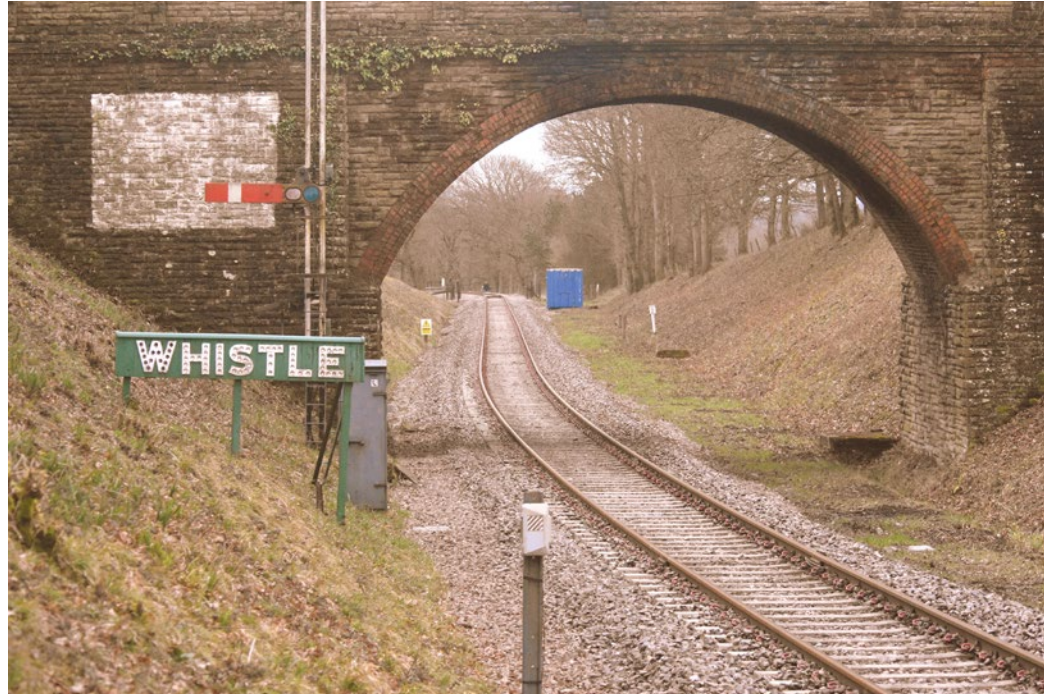
Horsted House Farm Bridge with finished replacement track, looking south towards Horsted Keynes. JON GOFF
