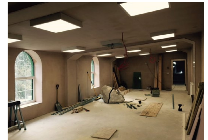
The first floor training room, with lighting and radiators installed, looking through to the new C&W office. ALL: STEVE BIGG
