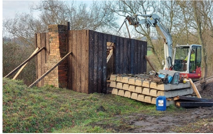
The Vaux End platelayers' hut being rebuilt around the old chimney. JON GOFF
