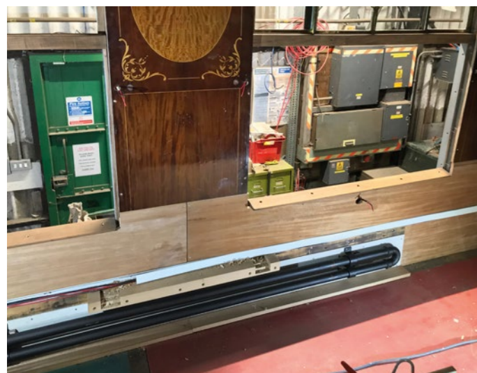
January 2021, and the steam heating, wiring for the attendant call buttons and table lamps are well advanced in Car No 54. RICHARD SALMON
