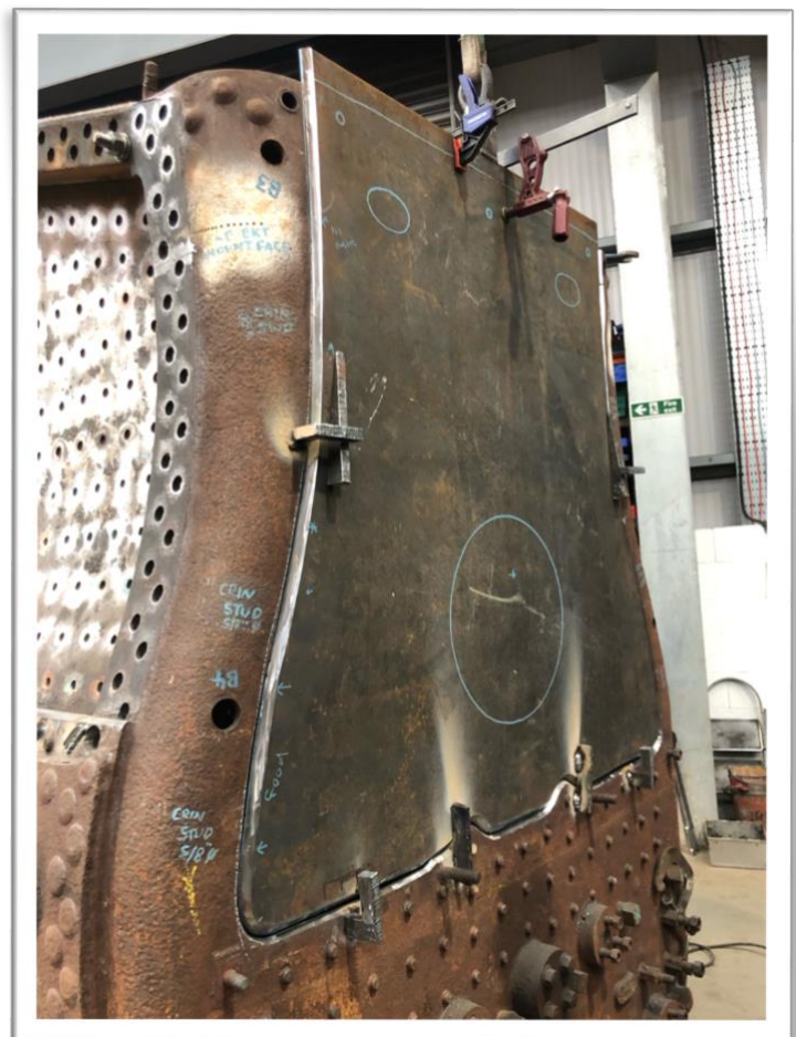
Top: New boiler plate awaiting welding into place on 541's firebox outer wrapper.
