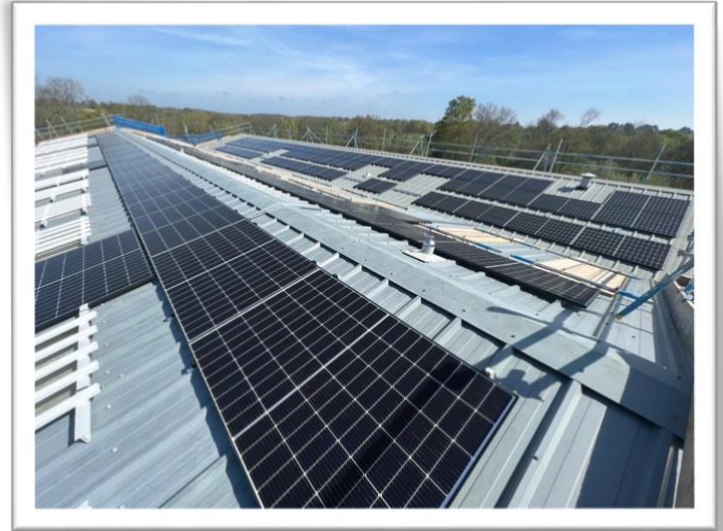
Above: A roof-level view of the new tiles. Photo courtesy of JoJu Solar
