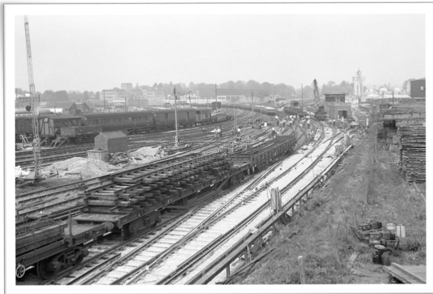
Left: [081868] Looking towards Horsham signal box during track relaying work, 9 May 1976. John Scrace
