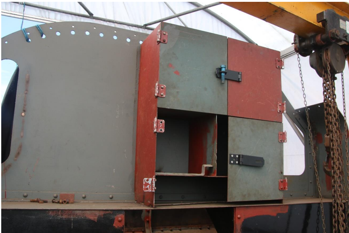
The tool box located on the bunker shelf has been constructed and welded in position. Three of the four doors have been fitted, and the wooden lining for the detonator storage in one of the compartments made.
