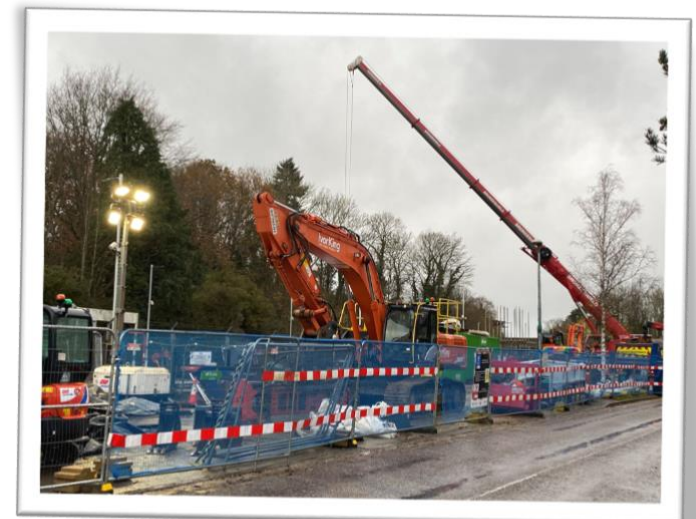
(Below) Two views of the construction work adjacent to the Bluebell station. Both photos: Roy Watts
