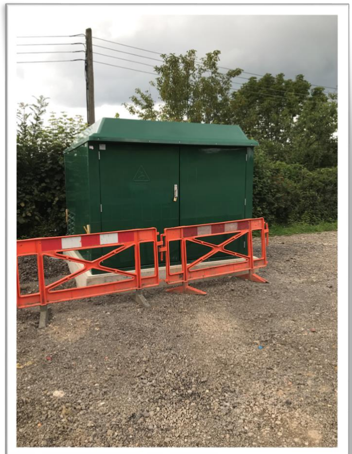
(Below) The new switching station
