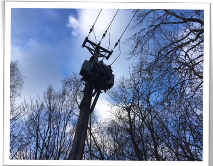
(Above) The existing 50kVA pole-mounted transformer
