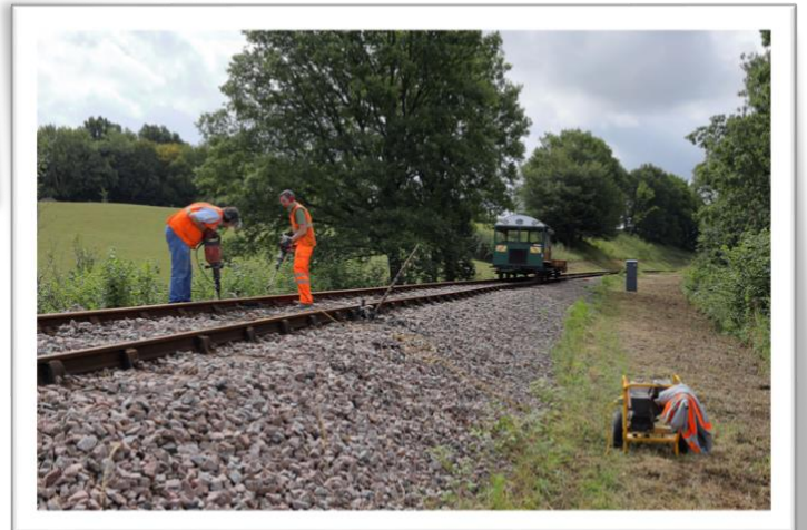
(Below) The Sunday Permanent way gang have also been back in action. One group, north of West Hoathly, were greasing fish plates and the second (pictured) were fettling the track alignment at Vaux End. Permanent Way work is one of the easier jobs to do whilst maintaining social distancing, outdoors. Photo: Dave Bowles
